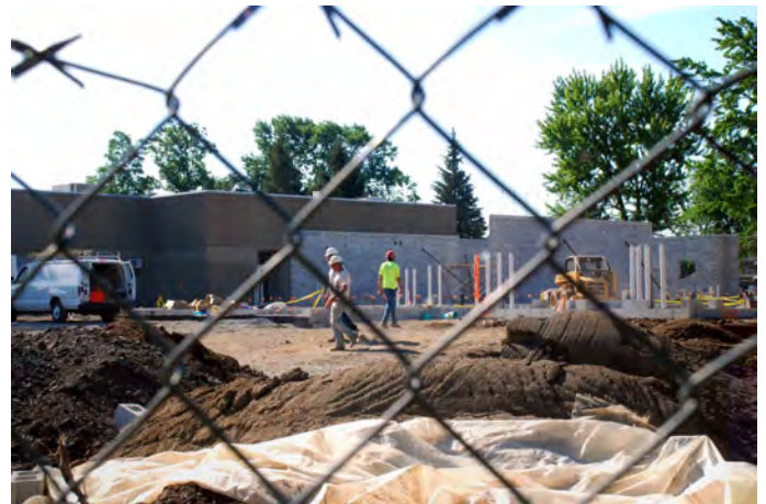
Progress is visible on the Davis Street Building addition, which has a finished foundation, and walls are being built.
