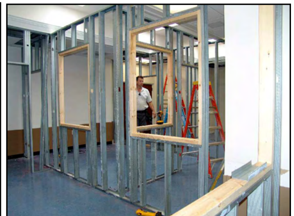
Left, the hallway on the second floor of the Village receives paint. Above, walls are framed for the new student media space. Photo credit: Mike Blinn
