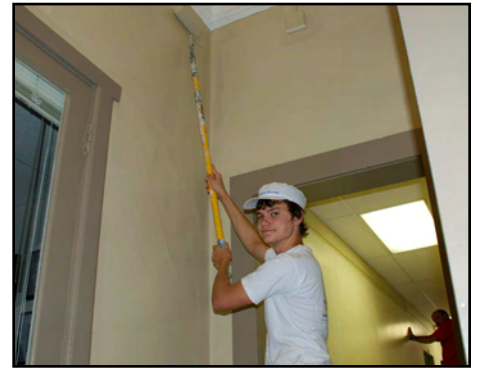
Mike Sears helps paint Old Main, which is just one of the buildings on campus receiving some renovations.
