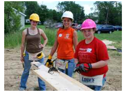
UF Habitat volunteers Heidi DeLong, Amber Daniels and Alicia Aldrich saw lumber for the new home.
