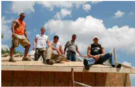
Justin Lyons, Scott Garman, Kevin McCann, Habitat crew leader Douglas Hipsher and Adam Snyder helped with roofing.
